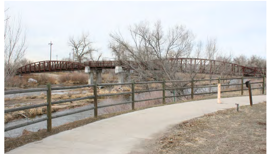
Looking northwest at pedestrian bridge over South Platte River in Fort Lupton
